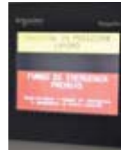
Check Control Panel
